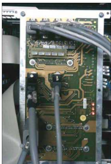
Fig 3.4 shows the position of the various trimmers on the RS012993.CSE board located at the rear of the electrical cabinet.
