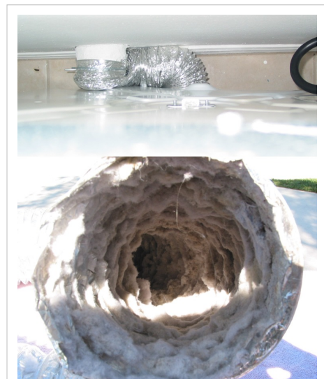
Upper image shows a severely kinked and blocked dryer transition hose used to vent a tumble dryer. In this case the dryer was located or pushed back too far against the wall. Lower image shows initial lint build-up in the flex transition hose.
