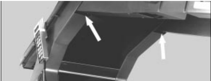
FIGURE 13 ..... Below Seat Joint Pinch Point
