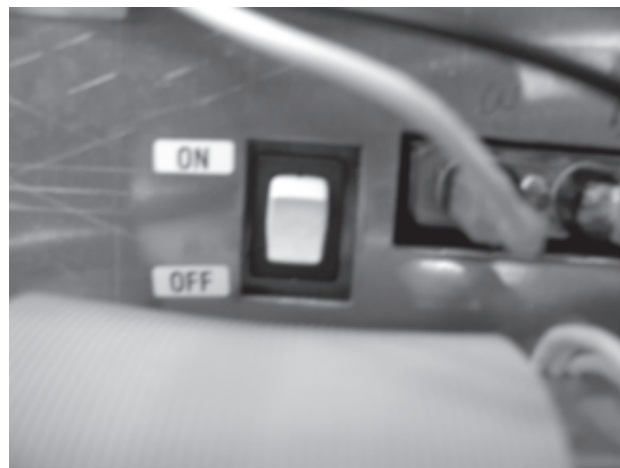
Figure 8-8. Harmony Wall Control ON/OFF Switch
